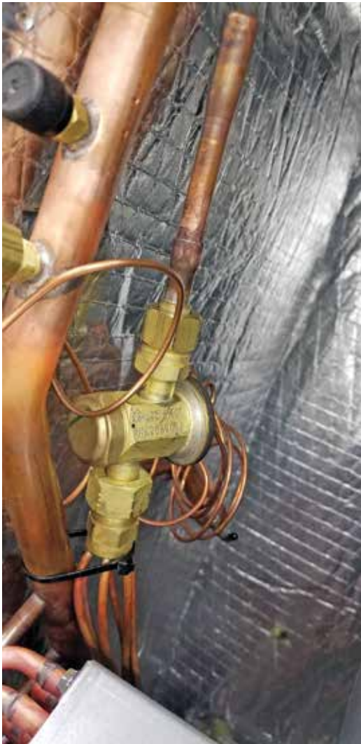
Figure 21: TXV Installed In Air Handler
